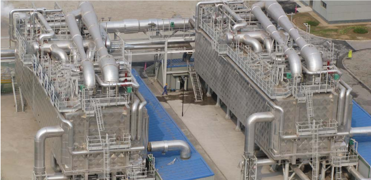
低温多效海水淡化主体装置俯瞰 Low temperature multi-effect sea water desalination main devices overlook
