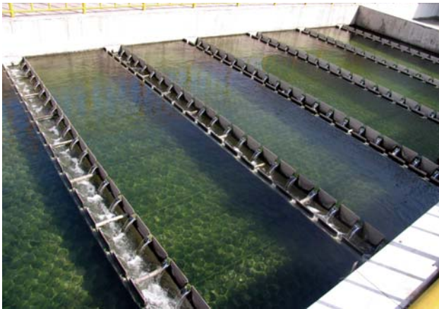
高效澄清池出水 Water Discharged by High-efficiency Clarifier
