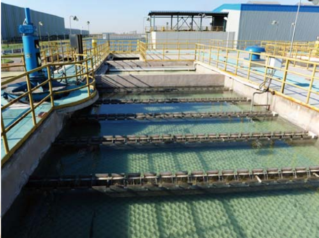
给水处理澄清池 Clarification pond for water supply
