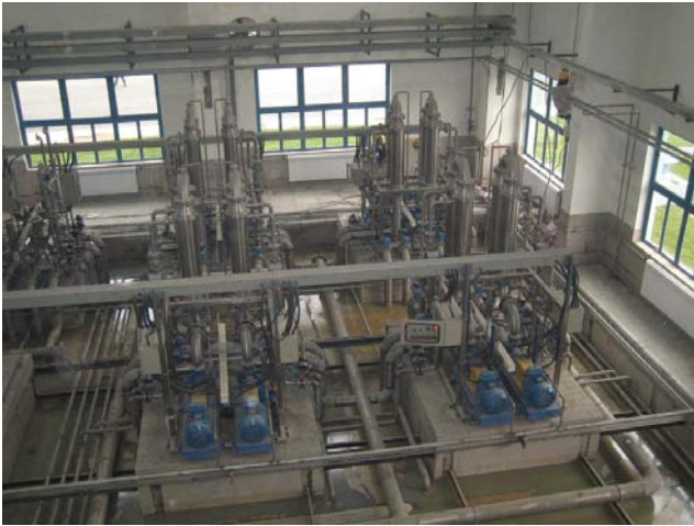
冷轧含油废水超滤布置 Arrangement of ultra filter for oily waste water from cold rolling mill
