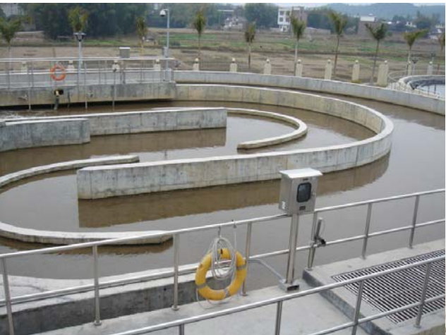
污水处理氧化沟 Oxidation ditch for waste water treatment
