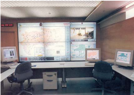
能源中心给排水管网计量与监控 Measurement and monitor system of water supply and drainage pipe network in the energy center
