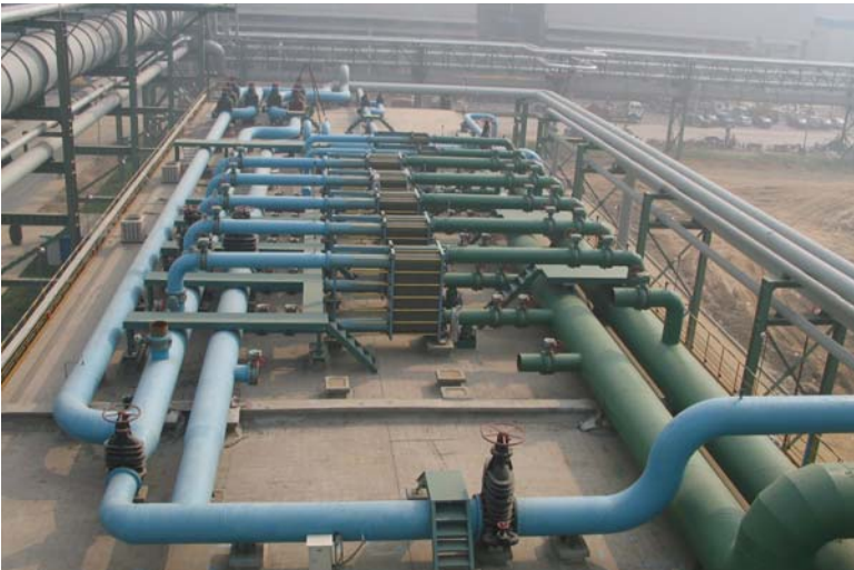
换热器局部 Part of heat exchanger
