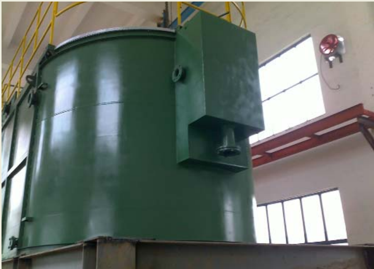
热轧含油废水一体化分离器 Integrated separator for hot mill oily waste water
