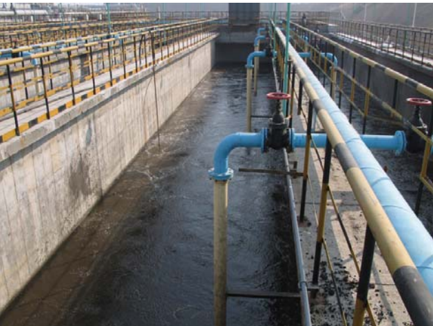
焦化污水处理生化池 Biochemical Pond for Coking Waste Water Treatment
