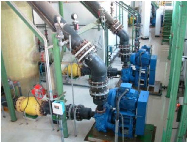
海水预处理循环砂泵房 Sea water pre-desalination circular sand pump house
