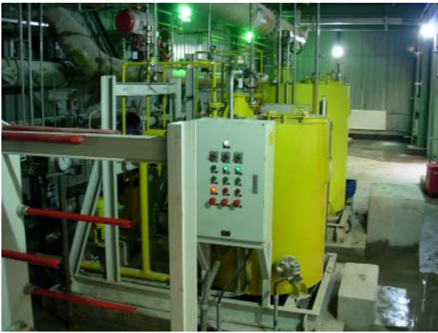
低温多效海水淡化辅助设施 Auxiliary devices for low temperature multi-effect sea water desalination project
