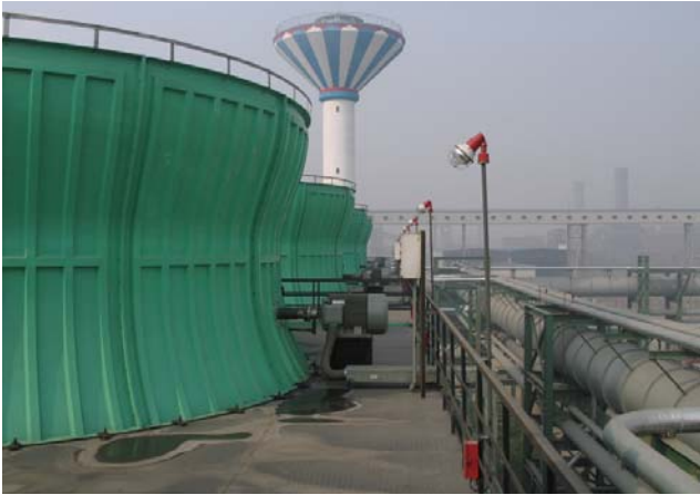
冷却塔及事故供水塔 Cooling tower and emergency water supply tower
